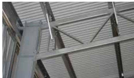
UB (Universal Beam) Columns - Big & very solid. And note the heavy fascia plate and roof truss to column plates. Bolted together with 8 x 20mm high tensile, grade 8.8 bolts makes this a super strong connection.
