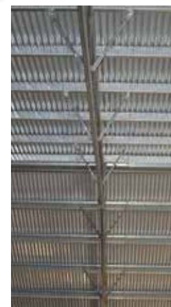
The flybraces that stop twisting of the roof truss in certain high wind, uplift conditions. This baby's not going anywhere!
